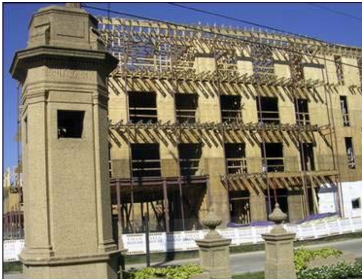
Work is under way on Fieldhouse, a New Orleans French Quarter-style condominium development just outside the pylon that marks the Nicholson Drive gates of LSU in Baton Rouge. The complex advertises that it is "600 yards from Tiger Stadium," provided that you take an angle and cut across parking lots. (Mike Hasten/The Times)
