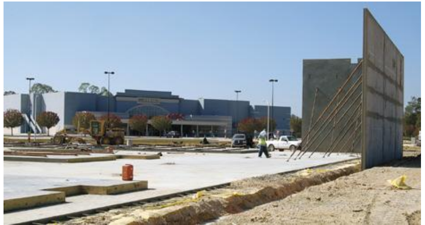
GOING UP — Workers install walls for the 127,380-square-foot Target store at Hammond Square on Wednesday. Photo by Joan Davis
