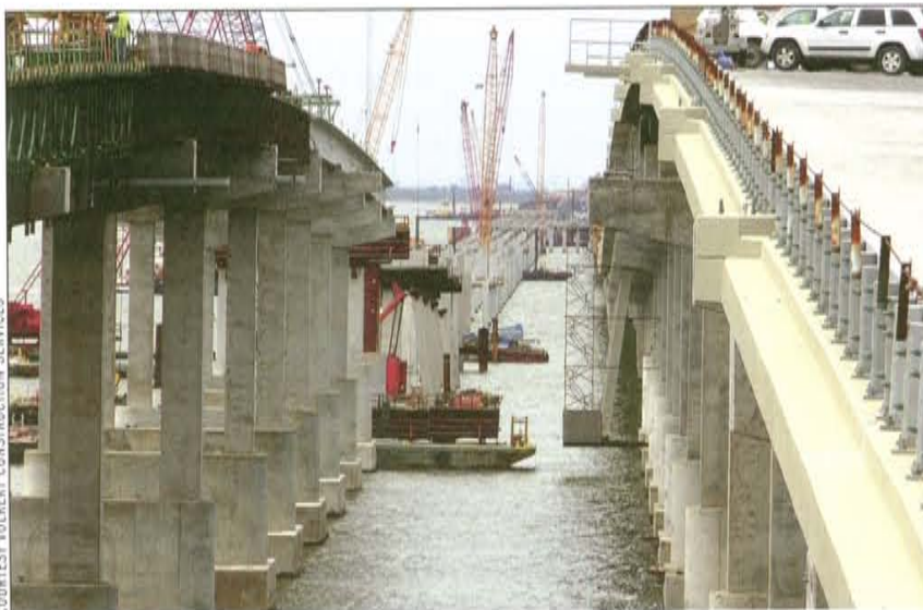
LAYING MILES: The largest projects in the region involve road construction—$1.2 billion to widen the Huey P. Long Bridge and $800 million to replace the I-10 Twin Spans.
