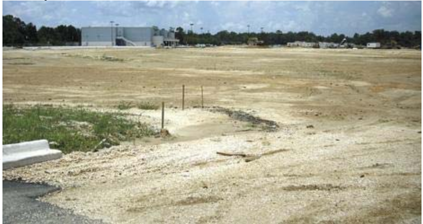
BIG AND WIDE —The smooth dirt surface is the future site of Target. at Hammond Square A traffic light will be placed at its intersection with U.S. 51.
