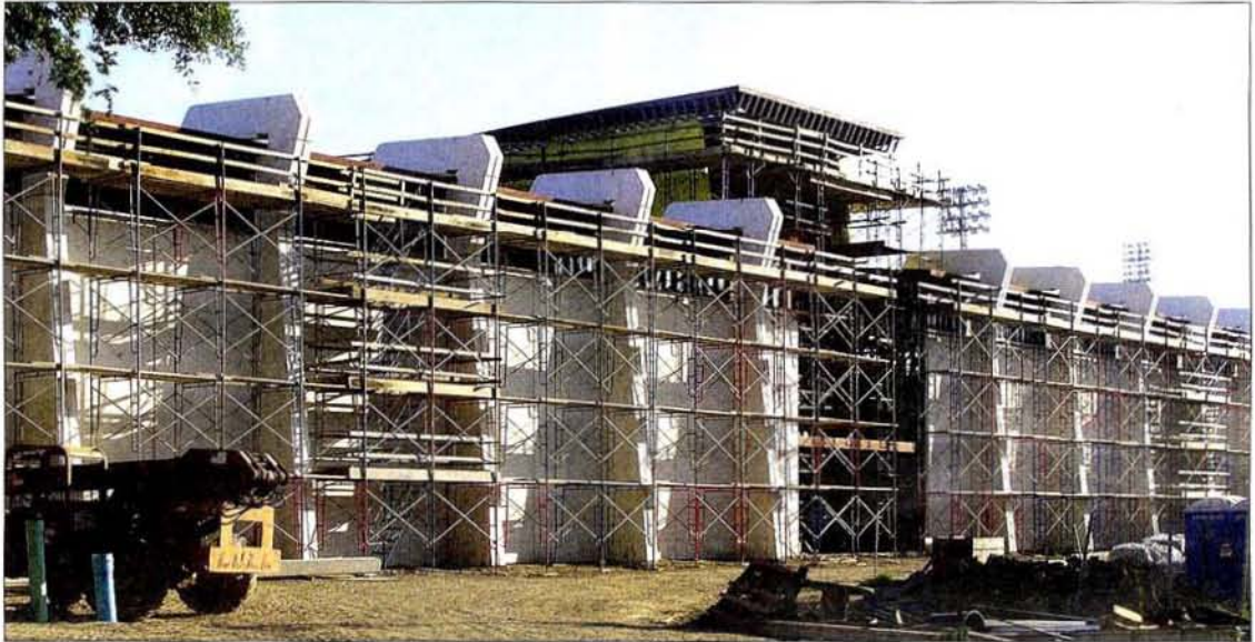
HOOP DREAMS: Construction continues on a $15 million addition to the Pete Maravich Assembly Center. The building, which will serve as a practice facility and locker room for the LSU men's and women's basketball teams, is scheduled to open for the 2009-10 season. Holden Architects/RDG designed the building, and Guy Hopkins Construction is the contractor.
