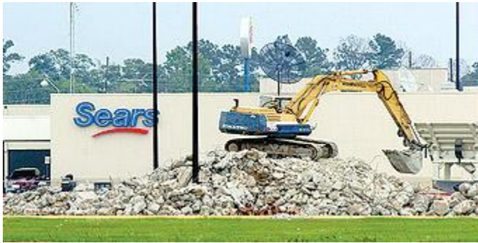
HILL OF RUBBLE – A backhoe operates atop a pile of broken concrete at the Hammond Square Mall demolition site Monday afternoon. The concrete will be pulverized and recycled for use in redevelopment. Photo by Kari Wheeler
