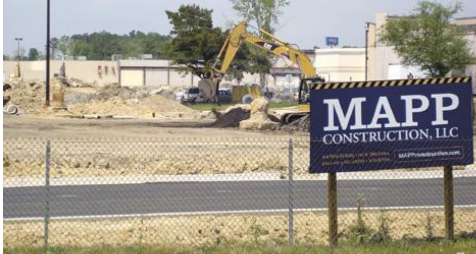
Viewed from Interstate 12, digging takes place Tuesday in the vicinity of Hammond Square where the Best Buy store will stand between Target and the soon-to-be expanded Dillard's.
