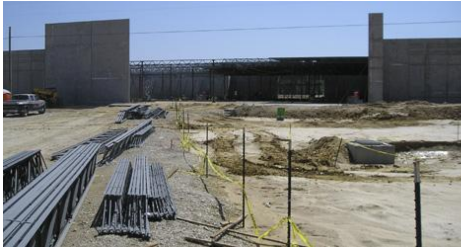
PENNEY'S — Walls for the new J.C. Penney retail store are going up at Hammond Square. Photo by Brennan David
