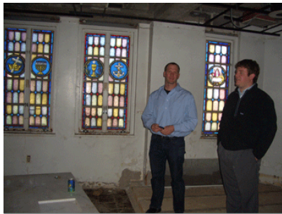
Reuben Teague of NOLA Community Development, left, and Barrett Cooper of Stirling Properties stand inside a former convent at 4230 S. Broad St. that could be converted into a gathering place for young professionals. (Photo by Emilie Bahr)
