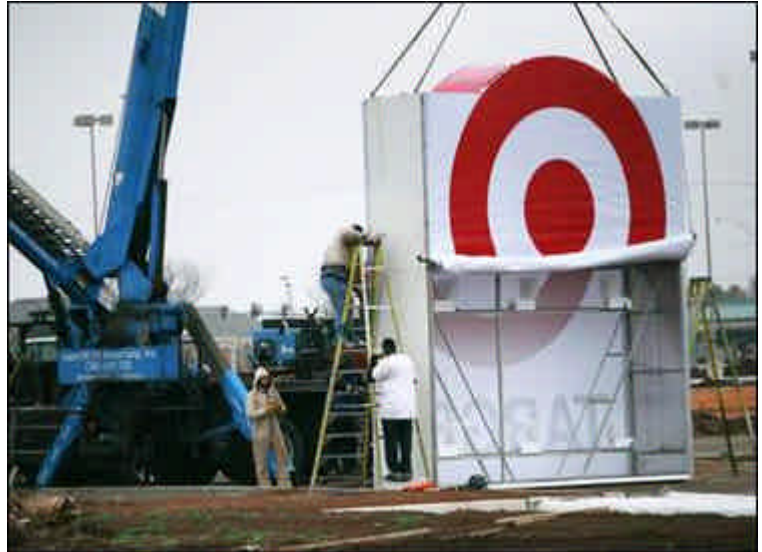
Workers prepare to erect the Super Target sign at the shopping center being built at Interstate 220 at Airline Drive in Bossier City. (Mike Silva/The Times)
